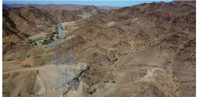
HANG2 transmission line | Arizona Public Service
