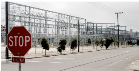
Pacific Gas and Electric substation. Bankrupted by high wholesale electricity costs during the 2000-01 Western Energy Crisis, PG&E is party to the ongoing proceedings related to market manipulation during the period.
